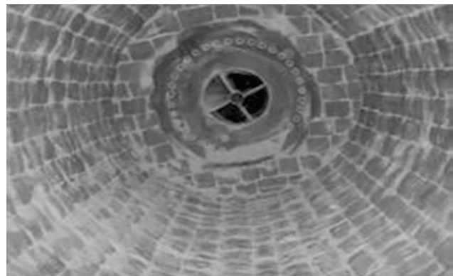
Figure 1. Snapshot of the interior of the industrial mill after the unloading process.
