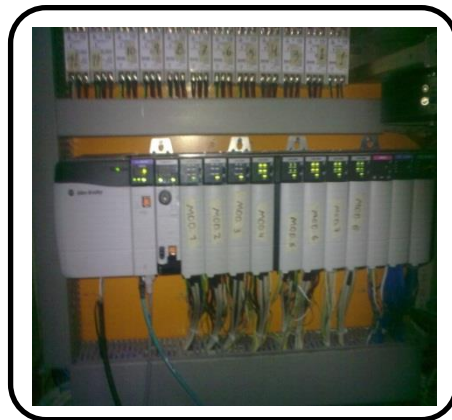
Figura 13. PLC Allen Bradley
